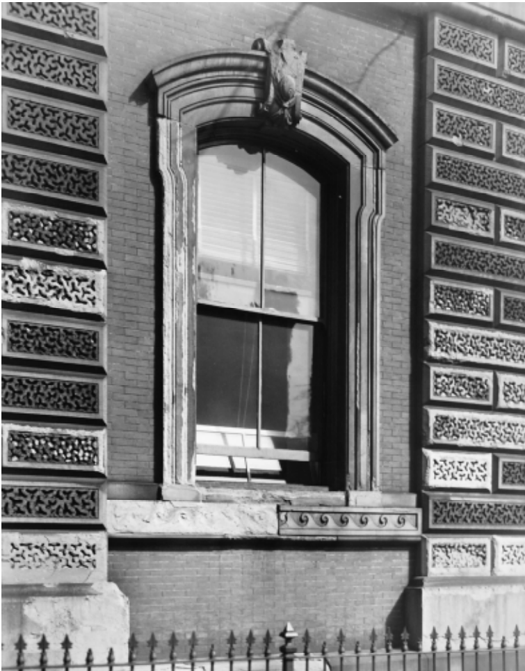
Photograph detailing crumbling sandstone, ca 1920-59 by Theodor Horydczak
